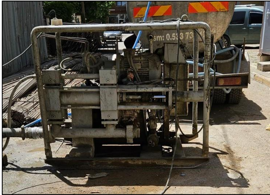
Figure 3.7 Jet Grout High-Pressure Pump Unit
