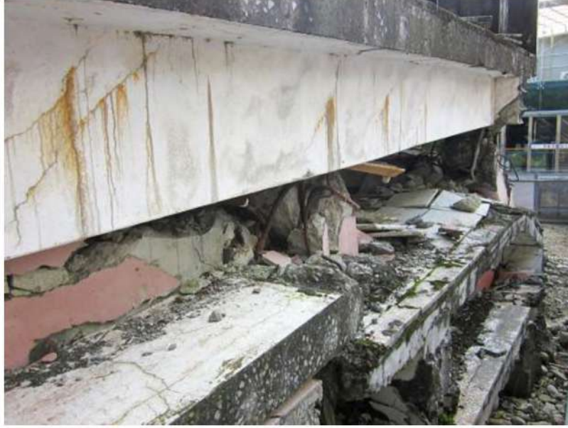
Şekil 3.10 Collapsed classrooms, are preserved at the 921 (Evans, 2013)
