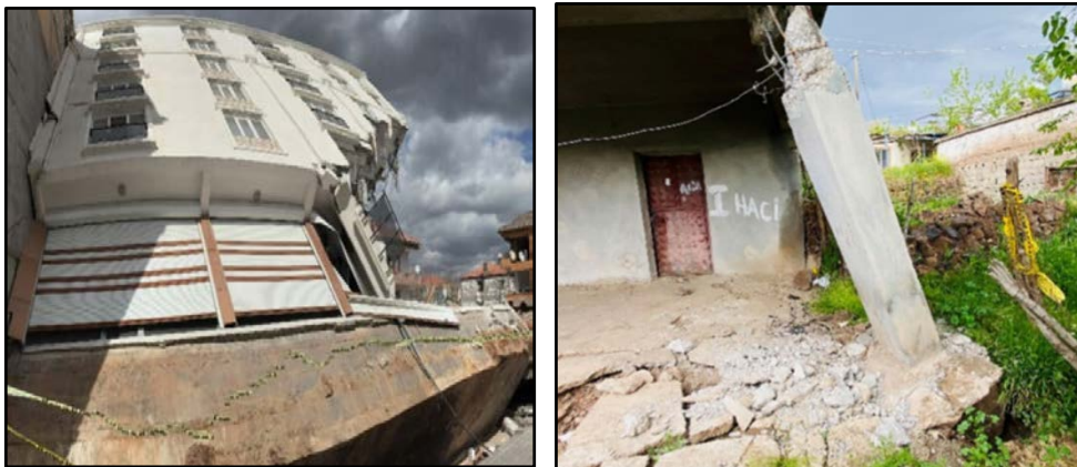
Figure 3.11 Damages arose from the Soil and Foundation system (Yön et al., 2024)
