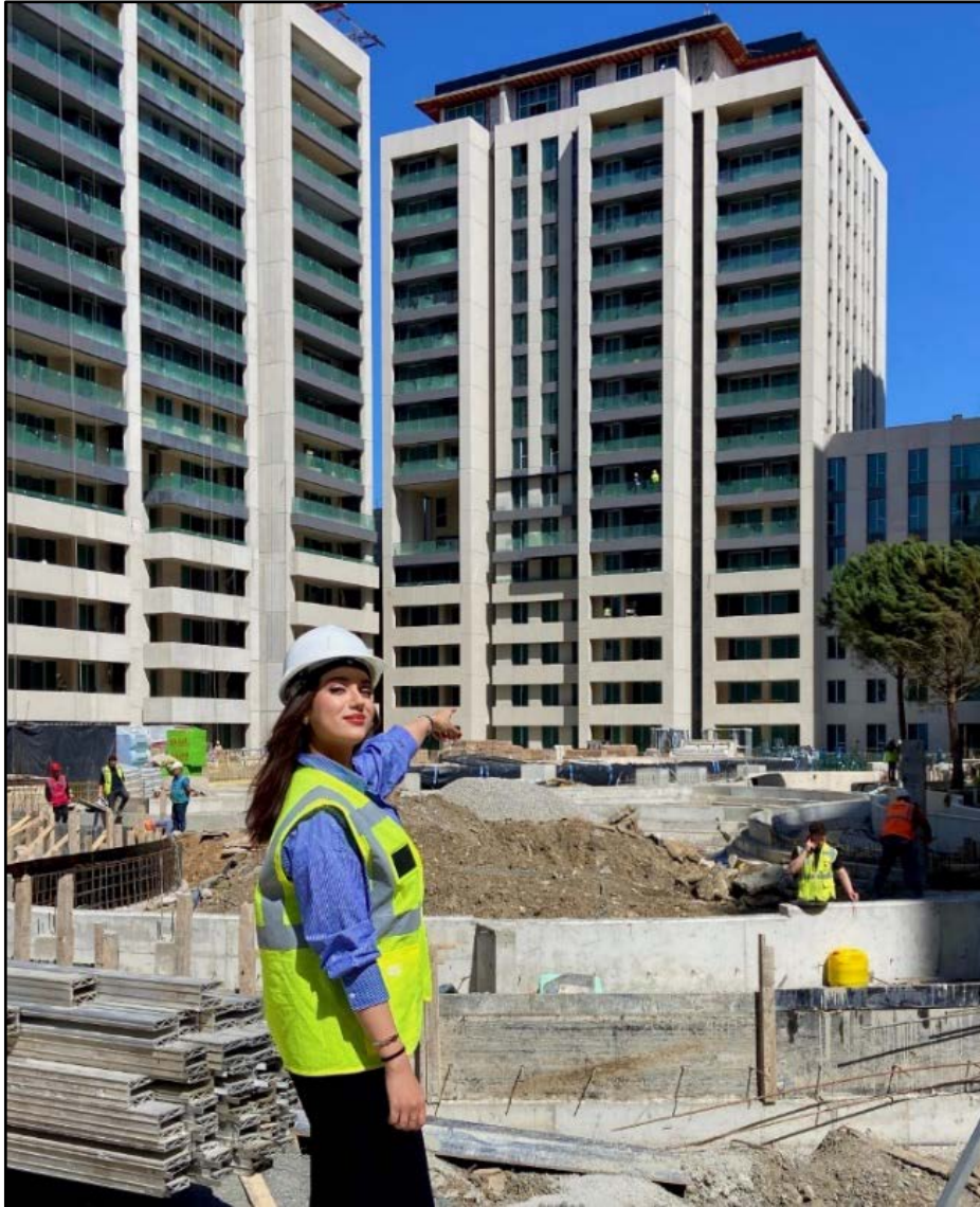
Figure 5.3 Front View Of Block A4 Chosen For Case Study From Site Of Construction
